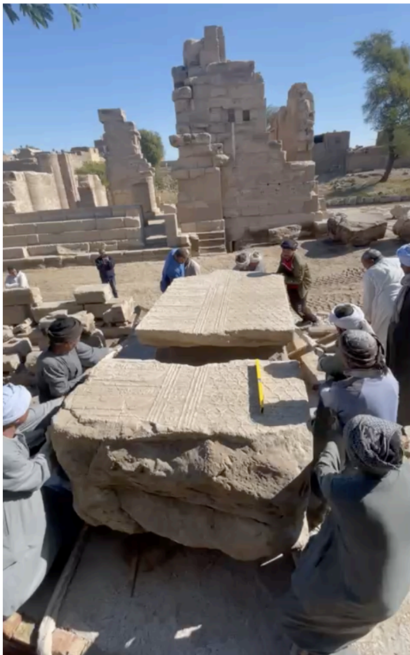
Skilled local workers reunite broken pieces of a massive decorated temple block atop the newly build display platform following conservation..
