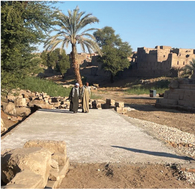
The newly built display platform that will keep the loose temple blocks off of the ground and protect them from groundwater, salts, and plants.
